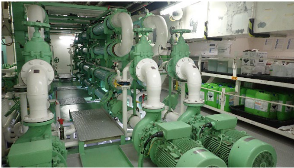
Wastewater treatment membrane bank
