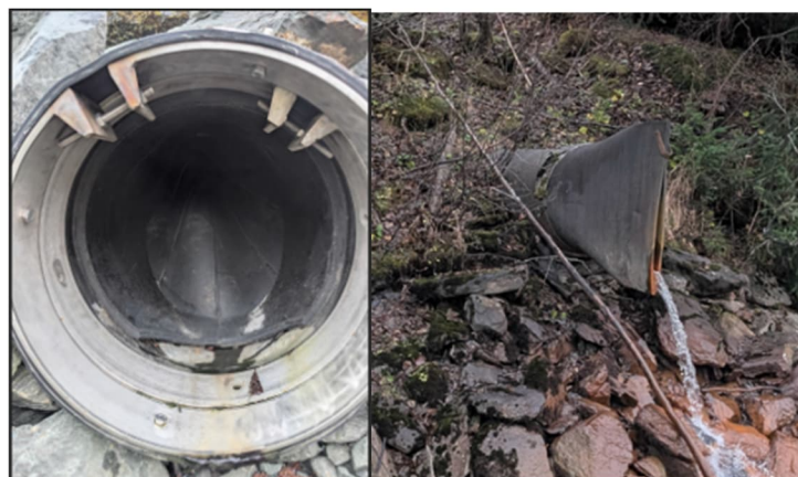
Figure 4-30 Backflow Preventors Currently Installed in Riverbank Drain Pipes (Rubber Gaskets Allow Stormwater from Protected Side Out, But Do Not Allow Water In)
