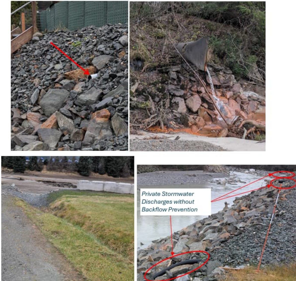
Figure 4-36 Photographs of Varied Drainage Outlets throughout the System that Would Require Reconfiguration/New Structures
