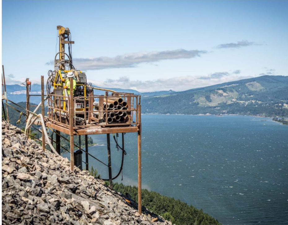
Figure 4-13 An Example of “Crux” Platform Installed on a Mountain Side
