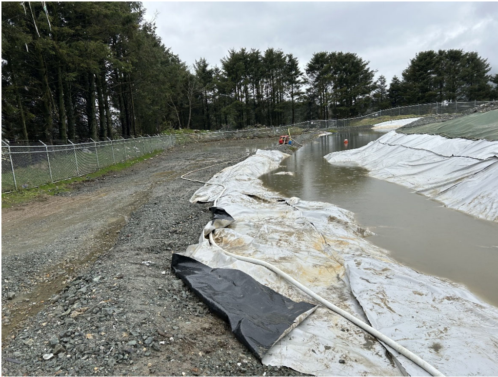
Figure 9. Stormwater is diverted onto perimeter road on the left of the picture. Lined leachate pond is on the right of the picture. Stormwater and leachate are pumped into municipal wastewater collection system at this time.
