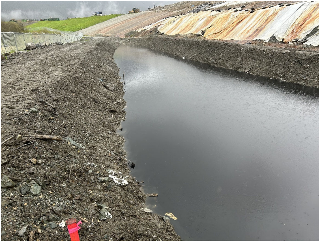
Figure 7. WM built an expansion area for the leachate detention pond that was unlined and therefore not approved by ADEC.
