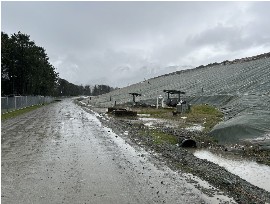
Figure 3. Stormwater infrastructure along the north east side of the landfill.
