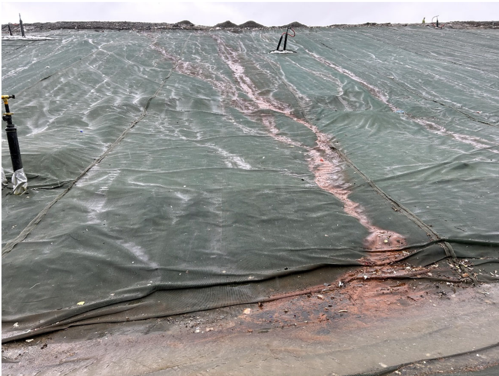
Figure 12. Apparent leachate seeps flowing directly into the stormwater system over intermediately closed waste.
