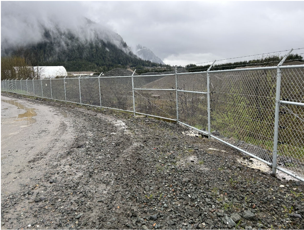
Figure 13. Perimeter bear fencing appears to be holding up well. Gaps beneath the fence are monitored and addressed as needed.
