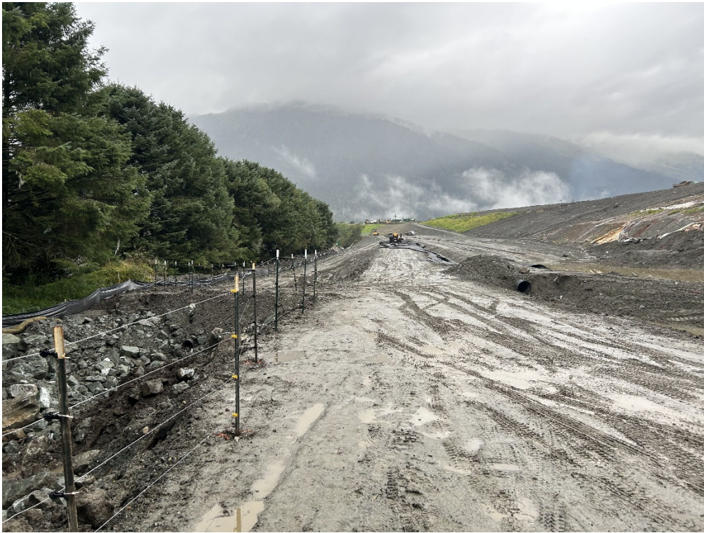
Figure 3. Temporary electric fence along the West Berm development of the landfill.
