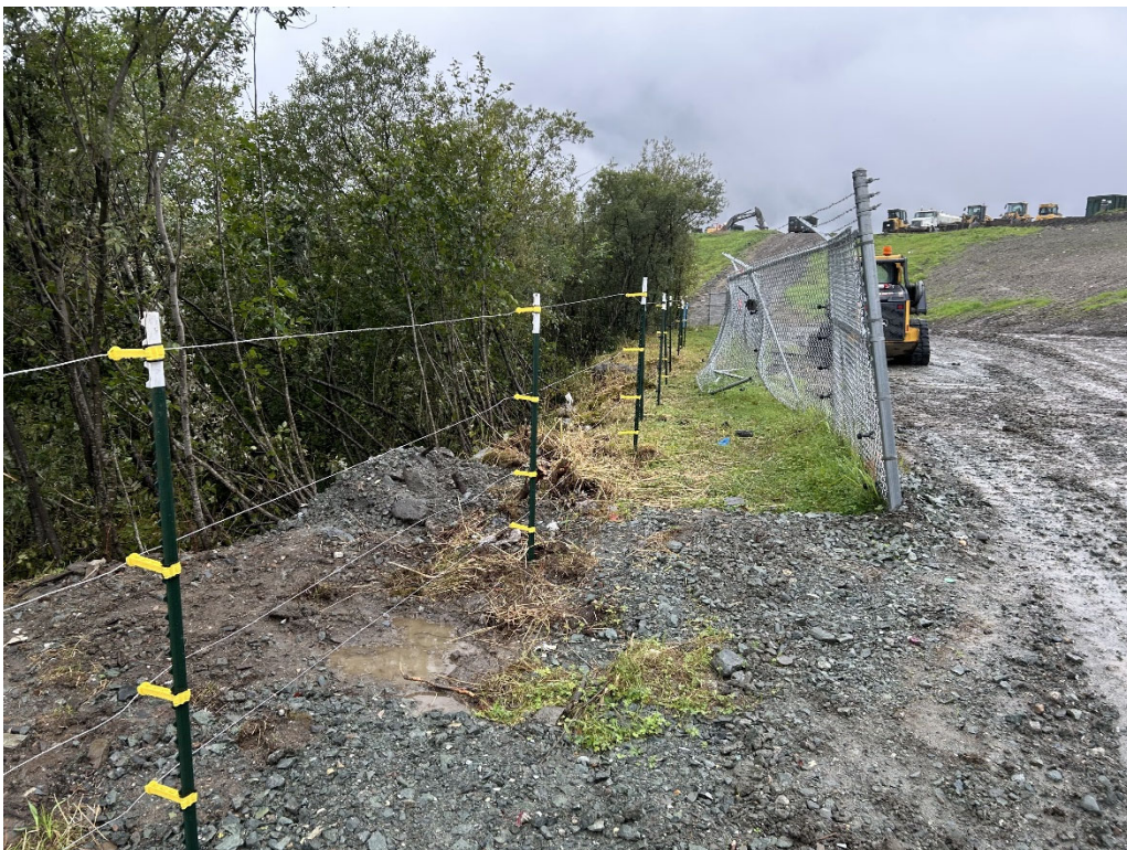
Figure 4. Temporary electric fence connected to the permanent perimeter fence; another game camera is present on the permanent fence.
